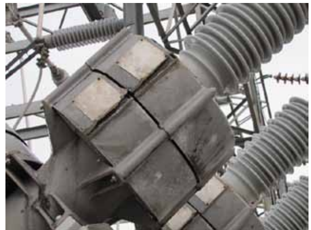
Cracked Outer Casing
